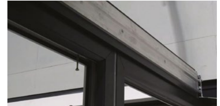
8 Fix the ringbeam to the window frames around the perimeter of the Skyroom roof.
