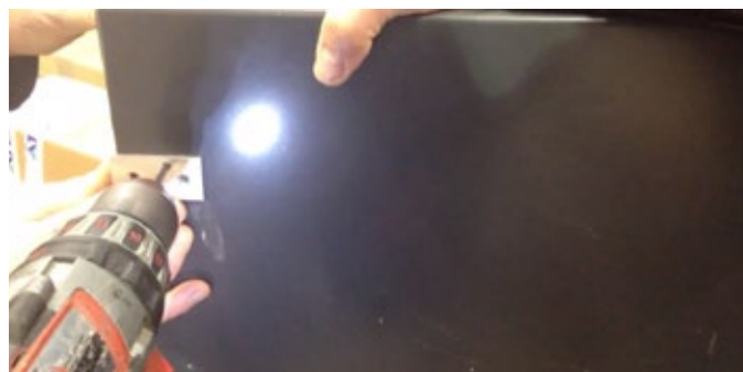
5 Use the cornice bracket again to drill the top 210mm hole right through the cornice.
