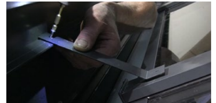
10 Fix the aluminium cornice support straps with screws from the top of the aluminium rafter cover cap to the back of the external cornice at each rafter.
