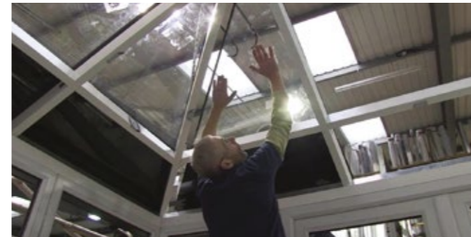
1 Glaze the remainder of the roof once all the upper ringbeams are fitted.
