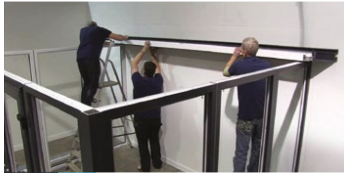
3 Lift the rear box gutter including the ringbeam and place it on top of the side window frames.
